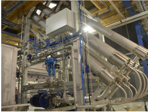
Figure 5: Ammonium sulphate by VP-Hobe Manure Valorisation system (ID 1529)
