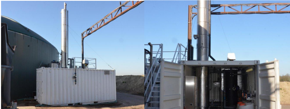
Fig. 2 Example of pilot installation in the Netherlands.
