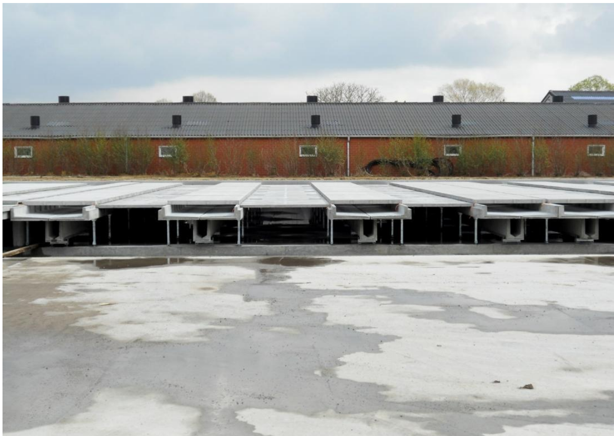
Figure 1. Plant for N recovery as urine from pig manure with "VeDoWS" adapted stable construction system.
